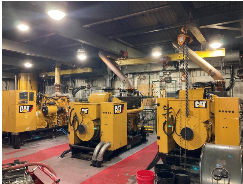
Figure 1: Mary's Harbour Diesel Generating Station
