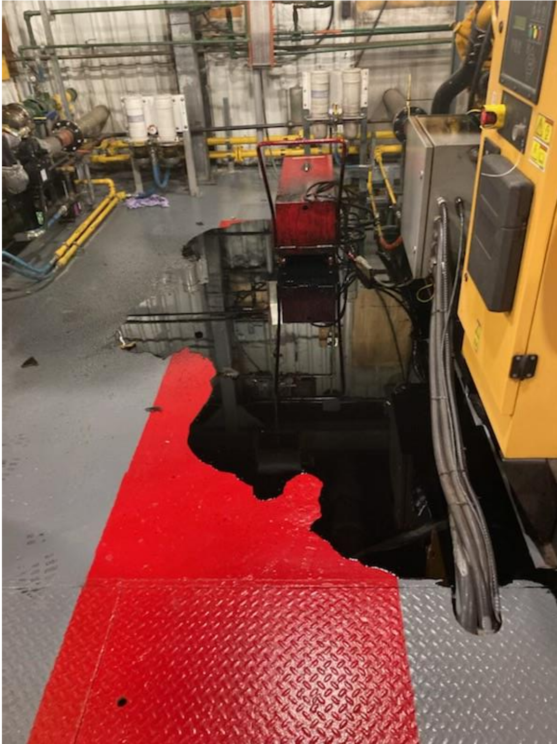
Figure A-3: Oil Spilled from Engine, due to Holes in the Engine Block, which was contained and remediated.
