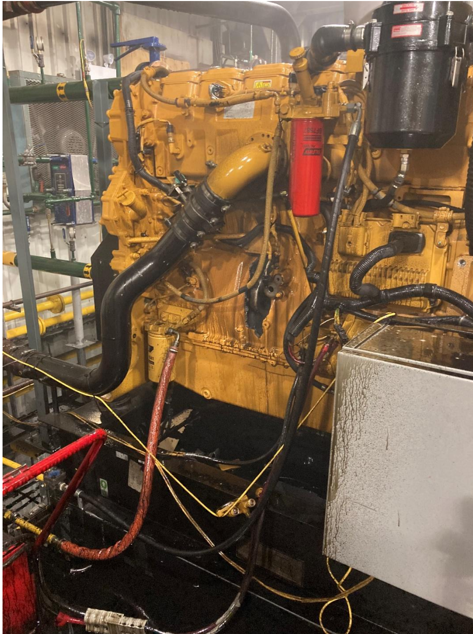
Figure A-1: Unit 2093 with Damaged Engine Block and Oil Spilled on Floor
